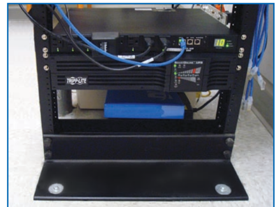
Miller relies on a Tripp Lite UPS System to provide a stable backup solution at each of their branch locations in order to protect Integra’s business-critical network.
